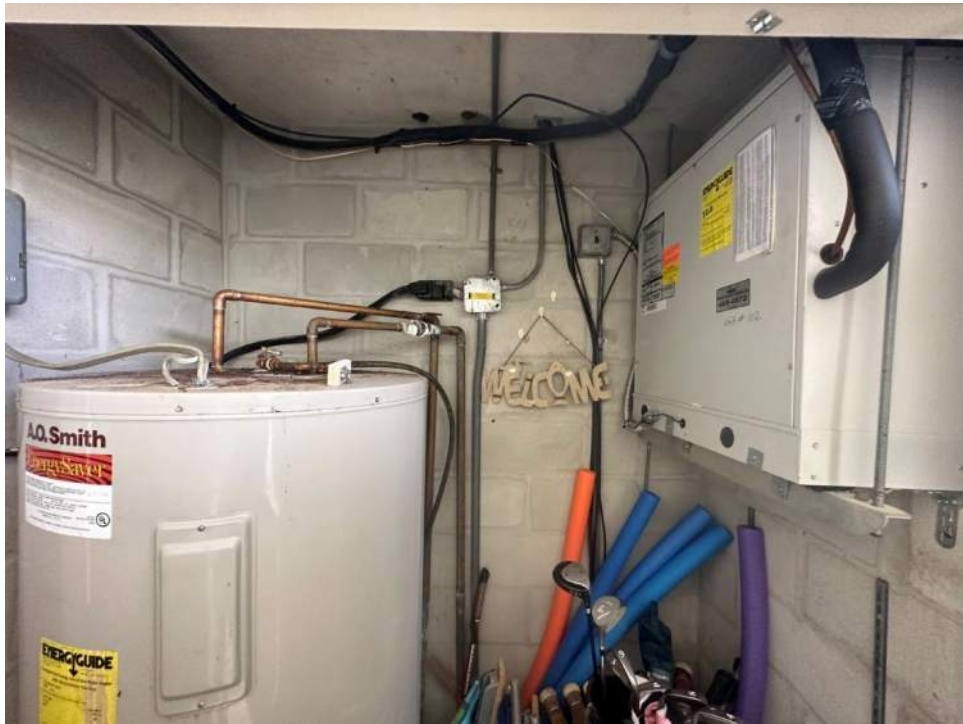
Figure 8: Water Heater Room
