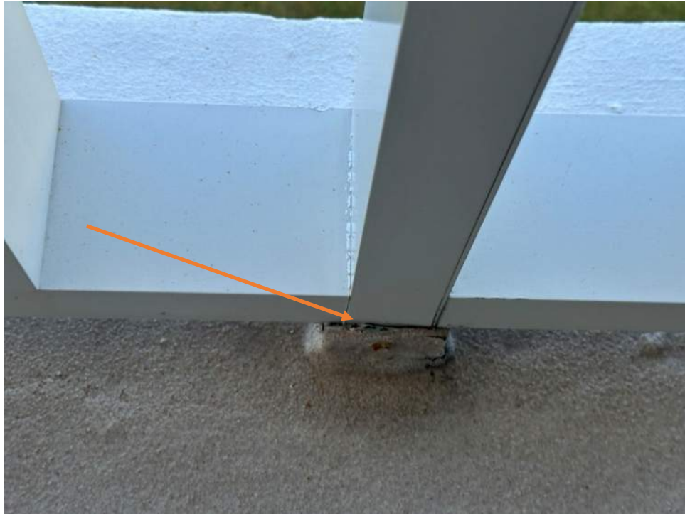
Figure 11: Deterioration at Guardrail Post Connection
